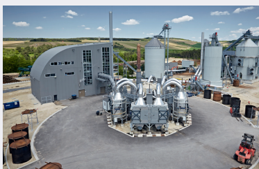
Cogeneration plant at Gyé-sur-Seine with pyrolysis kilns and wood-drying silos behind on the right.
