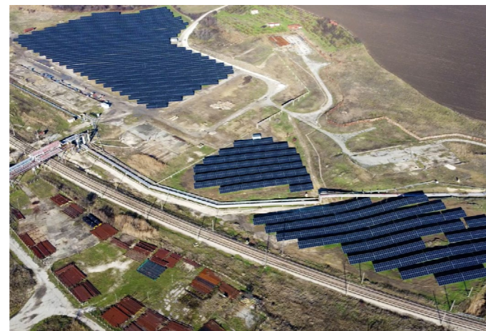
©GreenYellow. Solway solar power plant in Bulgaria with a capacity of 4 MW and an annual production of 5.3 GWh of green energy.
