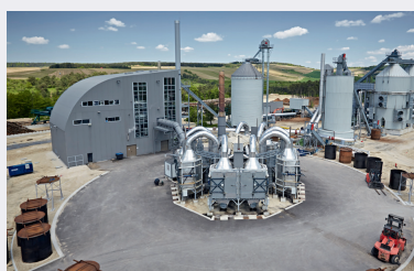
Cogeneration plant at Gyé-sur-Seine with pyrolysis kilns and wood-drying silos behind on the right.
