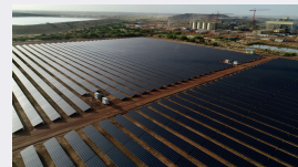
Essakane Solar, a 15 MWc solar power station commissioned in 2018 in Burkina Faso and serving the Essakane gold mine.
