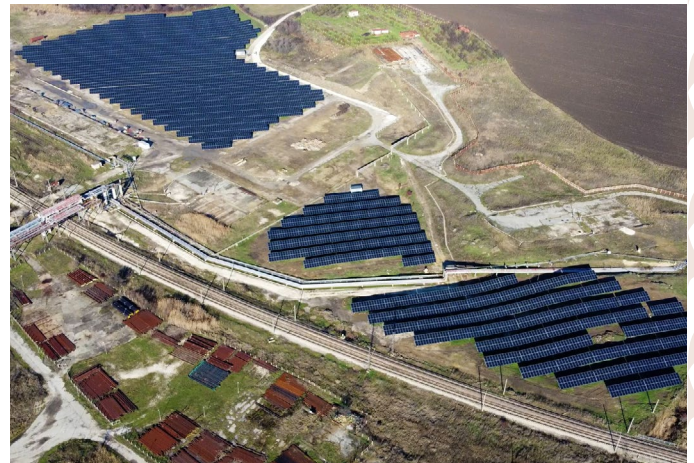
©GreenYellow. Solway solar power plant in Bulgaria with a capacity of 4 MW and an annual production of 5.3 GWh of green energy.
